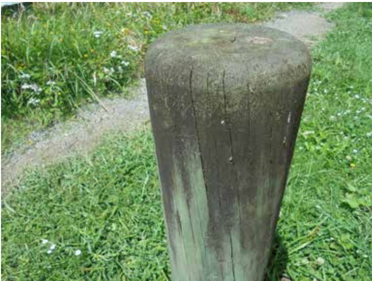
H-4 Treated Post: Structurally unaffected by Surface Mould
